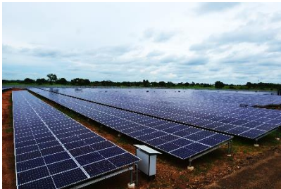
Kasim Textile Mill solar installation
