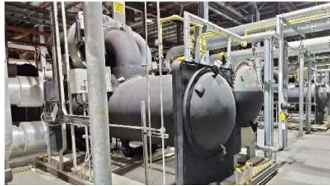
Chiller optimization at REC in Singapore
